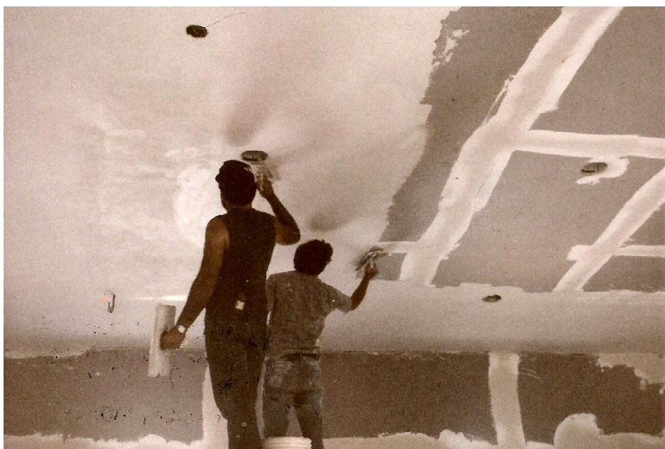
Two Men skim coat the arched ceiling in the upper level of the Historic Town Hall Would anyone know the identities of these men? Boylston Historical Society Photograph Collection
